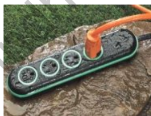
Fig: 15.24 Electrical extension placed damped environment
