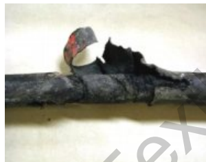
Fig: 15.23 Over heating of a cable
