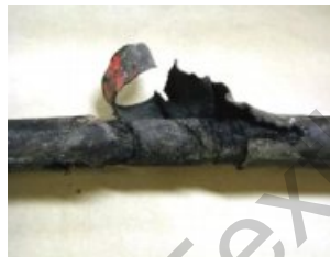
Fig: 15.23 Over heating of a cable
