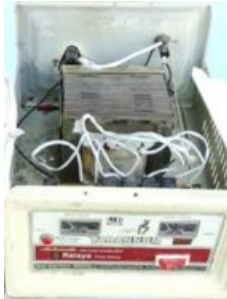
Fig: 16.20 Transformer in stabilizer
