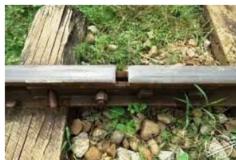
Fig 9.13 Gaps between Rail Tracks
